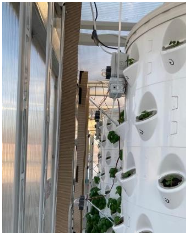
Figure 21 – Image of the LED control system installed at the farm
