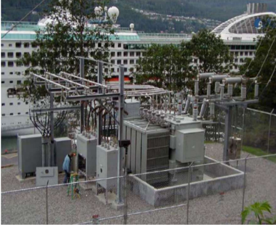
Figure 4 Dual Voltage Transformer to step down the voltage (Port of Juneau) [5]
