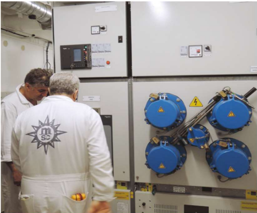
Figure 6 Ship connection point on Switchboard [15]
