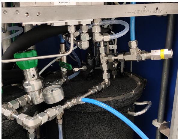
(a) Low pressure regulator and pressure relief valve
