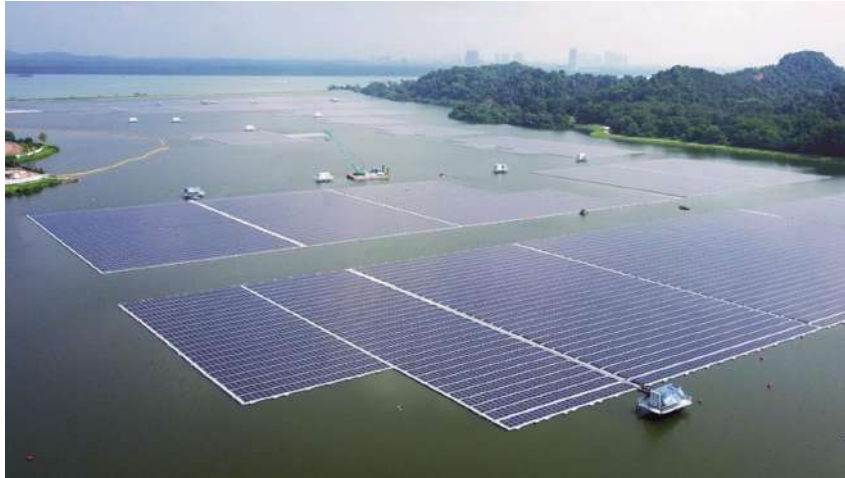
Figure 2.12: Floating System in Tengeh reservoir, Singapore.
