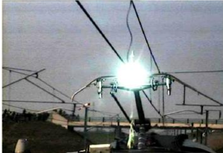
Figure 2.4: Arcing and dropper slacking in a standard railway vehicle operation
