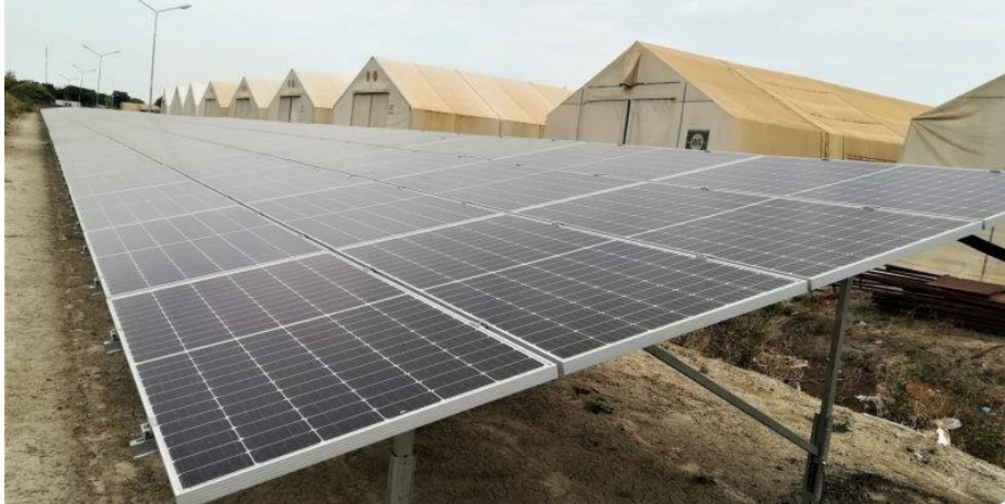
Fig 2.2 700 kWp Solar photovoltaic system in Malakal, Upper Nile State in South Sudan. [ https://www.afrik21.africa ]
