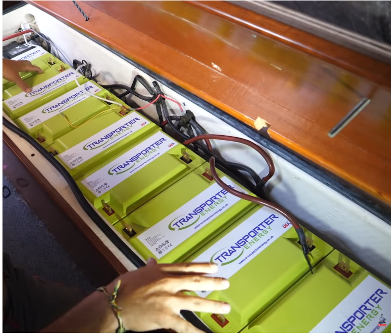
Figure 5.5: SV Delos - Lithium battery pack.
