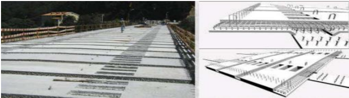
Figure 2.3 - Concreting of the deck of the Penacova Bridge over the Mondego River – use of pre-slabs [11]
