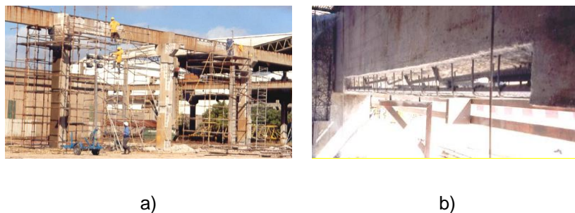
Figure 3 - Removal of concrete: a) with a pneumatic hammer; b) in the area involving the reinforcements
