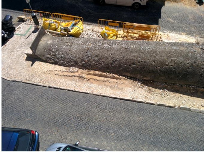
Figure 46- Pavement in very bad condition
