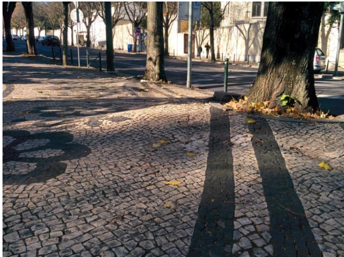
Figure 47- Pavement in Moderate Condition
