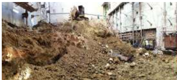
Figure 6 – Figure that illustrates the parallel execution of different levels of panels. The most delayed part of the excavation is near the entrance, in order to give access to materials and equipment.
