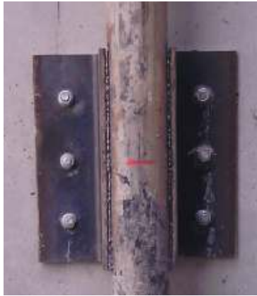
Figure 3 – Steel section guarantying the vertical forces mobilization between the retaining wall and the micropile.
