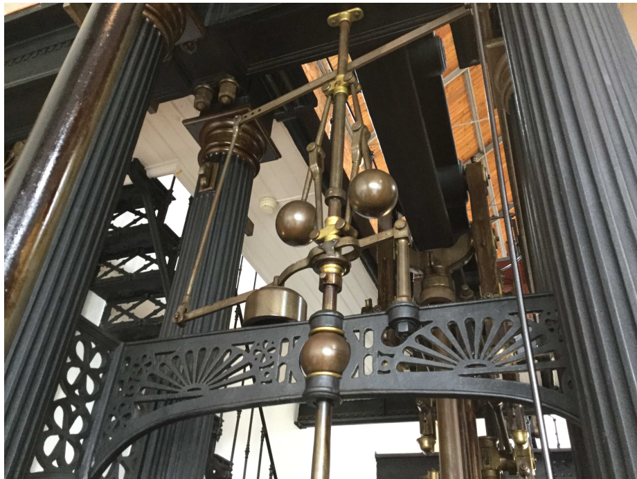
Figure 9.6: Centrifugal governor of a boiler in the former Barbadinhos water pumping station (currently the Water Museum), Lisbon.
