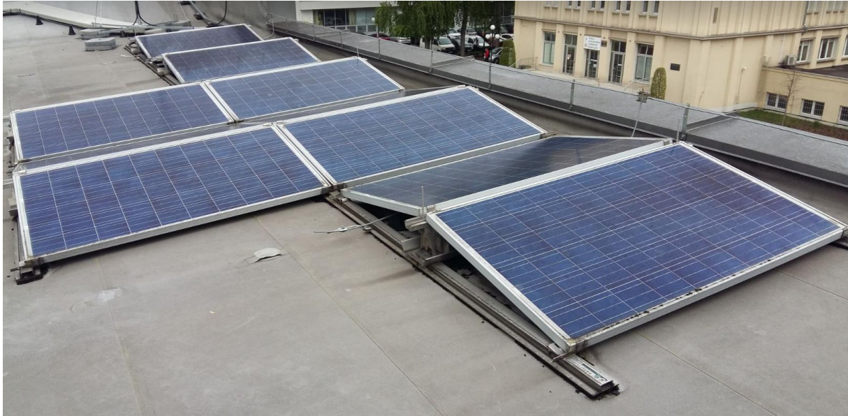
Figure 5. Solar panels at AGH UST in Cracow, Poland
