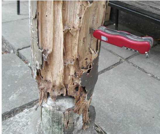
Figure 13- Significant termite damage to bamboo column in Costa Rica (Kaminski, 2018).
