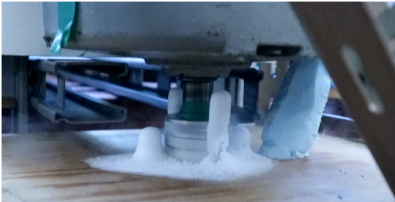
Figure 4.6: Ice build up in the coupler surroundings
