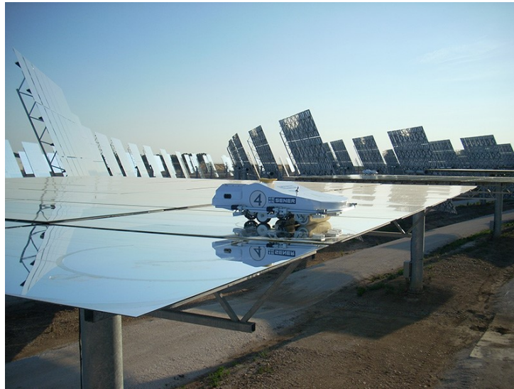
Figure 2.2: Heliostat cleaning with HECTOR at the Gemasolar solar power plant [29].
