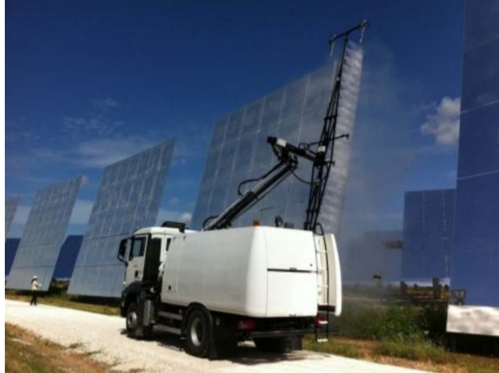
Figure 2.1: Traditional heliostat cleaning approach using high pressure water and large hydraulic arm [19].
