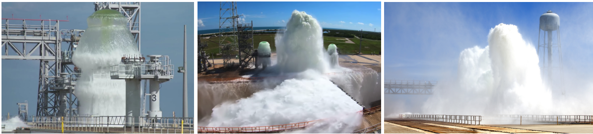
Figure 1.3: SLS water acoustic suppression system. [3]
