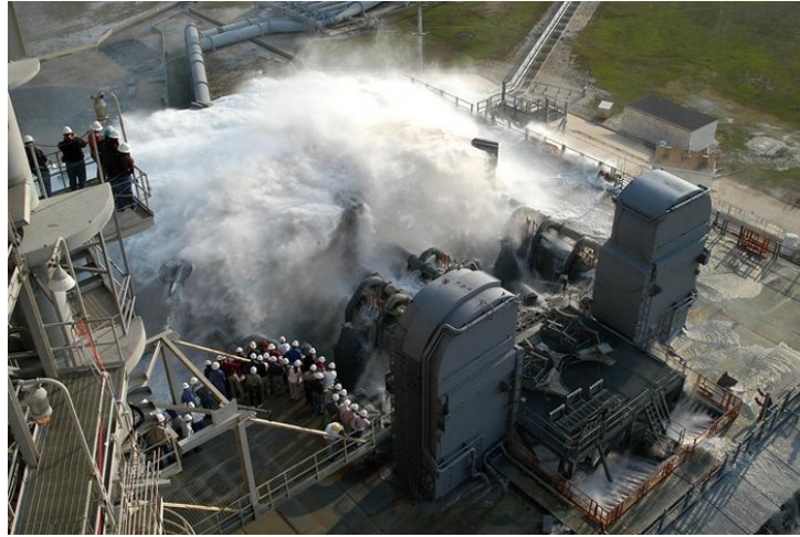
Figure 1.2: Space Shuttle water acoustic suppression system. [3]
