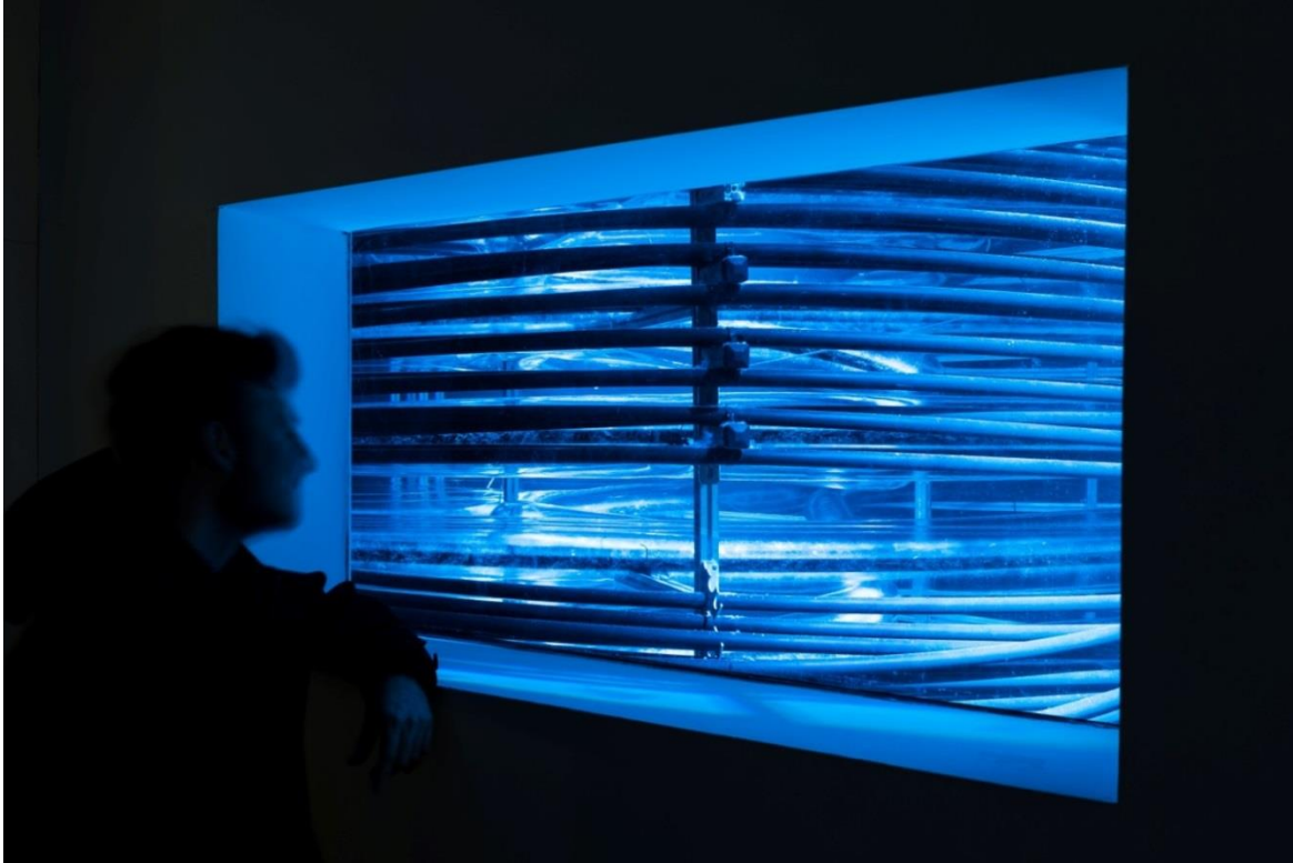
Figure 13: Ice Storage Regeneration Heat Exchangers (Source: Audio Tuning Vertriebs GmbH)
