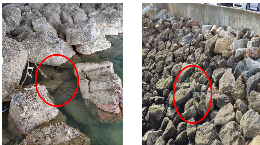
Figure 1 - Slabs in different environmental exposure conditions XS2 (left) and XS3 (right)
