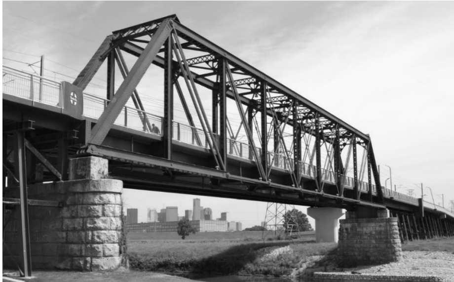
Figure 4.3 - A Third Example of a Metallic Bridge, Santa Fe (extracted from [Fell13]).
