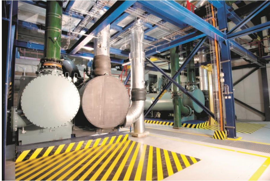
Figure 3.3 Centrifugal chillers of Climaespaço Plant [33]
