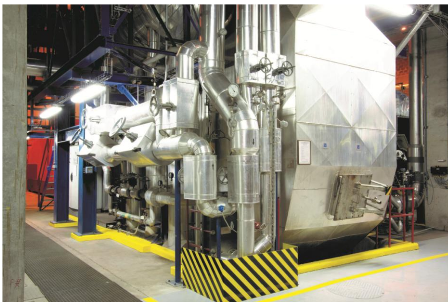
Figure 3.1 Heat recovery boiler of Climaespço Plant [33]
