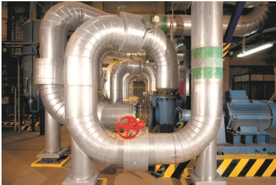
Figure 3.2 Distribution pipes of Climaespaço Plant [33]
