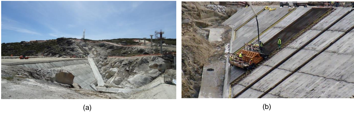
Figure 1: Montesiinho Dam: (a) rockfill embankment construction; (b) curtain construction with slip form.
