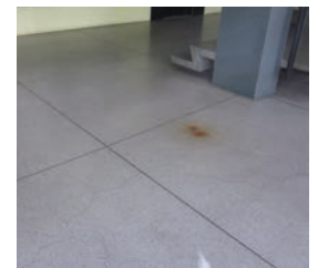
136. Cracks and spots on the inner terrazzo flooring. Hall Calas . (April 4 th 2014).
