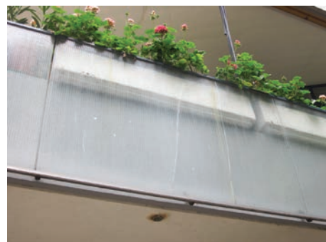
174. 175. Wired glass is also used in Miremont-le-Crêt as a covering panel of the reinforced concrete parapets - instead of the prefabricated concrete panels. Cracked panel (May 8 th 2014).
