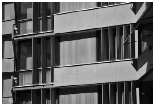
202. View of the façade of the building A in the end of the rehabilitation works (Meier+associés architectes).
