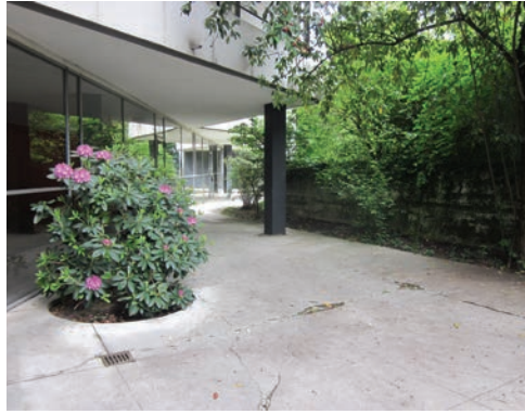
139. Several cracks and fragments on the exterior flooring. Outside the Calas' hall (May 8 th 2014).
