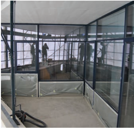
199. New fibre cement panels protected during the final painting of the window frames (May 26 th 2014).
