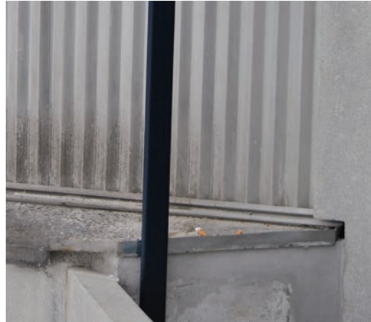
180. Deteriorated aluminium protecting drip (May 8 th 2014).
