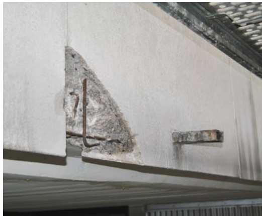
188. Carbonated prefabricated concrete panel (May 26 th 2014).
