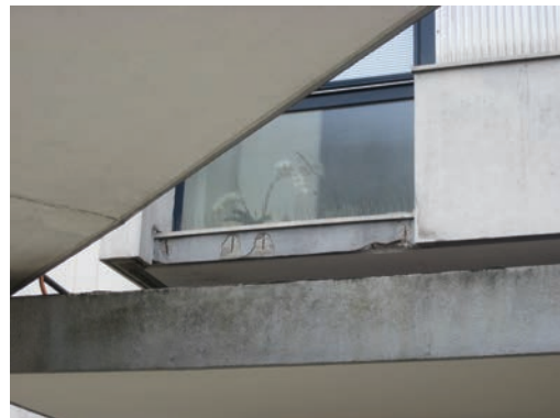
163. Carbonated concrete elements. Frameworks exposed to the air and corroded (May 8 th 2014).
