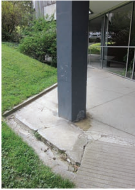
138. Cracks and fragments around a pillar (April 4 th 2014).
