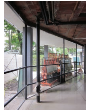
152. False columns dismantled during the rehabilitation works on the piping system. Miremont's hall (May 8 th 2014).
