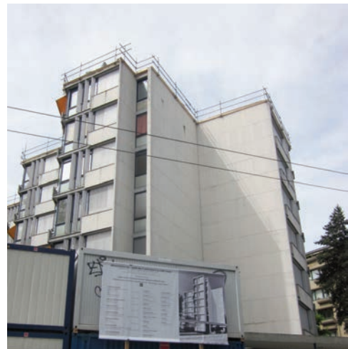
182. View of the gable-end façade. On top some of the prefabricated concrete panels are deteriorated (May 8 th 2014).
