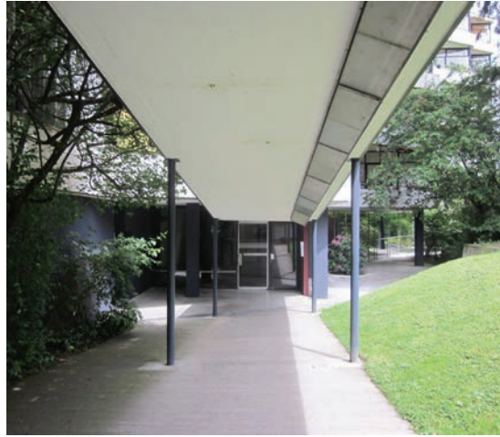
148. Lighting devices on the entrance on the side Calas . Moss under the breezeway (May 8 th 2014).
