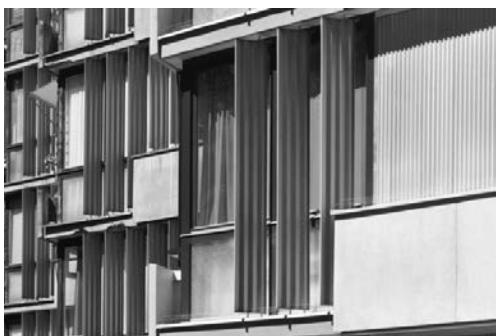
201. View of the façade of the building A in the end of the rehabilitation works (Meier+associés architectes).
