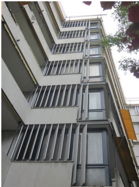
173. Wired glass parapets integrated in the window frames of the building’s façade (May 8 th 2014).
