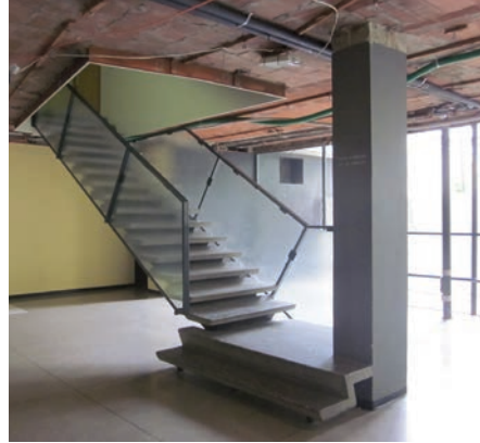
155. Condition of the staircases. Miremont's hall (May 8 th 2014).
