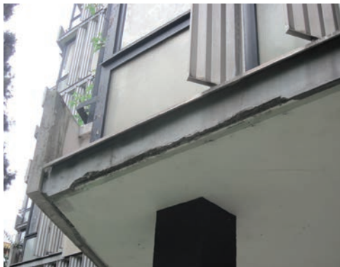
162. Carbonated concrete elements on the edges of the slabs (May 8 th 2014).
