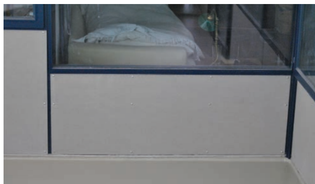
172. Balconies' renovated opaque parapets with new fibre cement panels (without asbestos) (May 26 th 2014).
