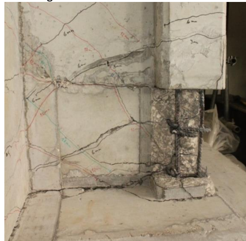
Figure 5.3 – Final cracking of V2 beam
