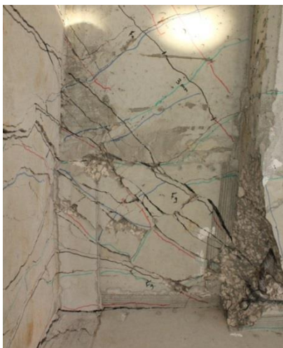
Figure 5.5 – Final cracking at V4 beam
