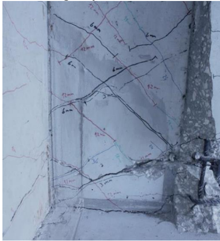
Figure 5.4 – Final cracking of V3 beam
