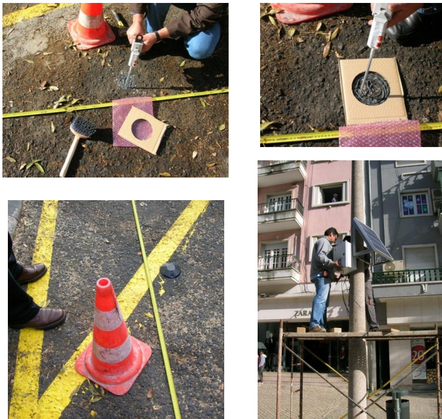
Figure 5.15 - On top: The two pictures show the glue where de sensor will be installed. On the bottom left we can see the sensor after being glued on the ground, and on the right it is the Gateway being installed, which is powered by a solar panel. Source: author
