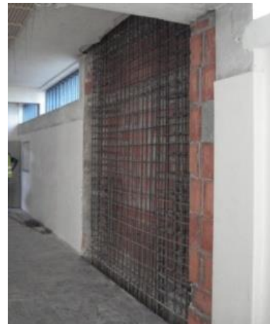
Figure 6 – Addition of shear walls in Leonor School (photo taken in 2010-10-25 by author)
