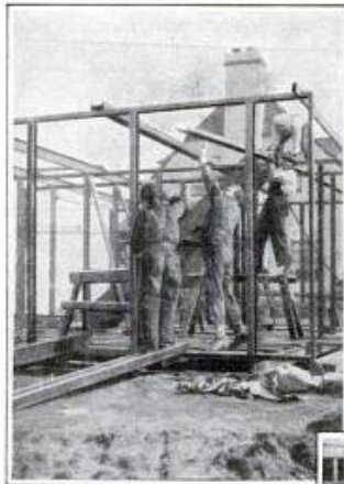
Erection of the steel framework of a house at Forest Hills, N. Y., in three hours and fifty minutes. The side framework being raised and bolted.
