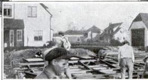
Checking over the steel material which a few hours later was a house, built as illustrated in the photographs above. The mate-
