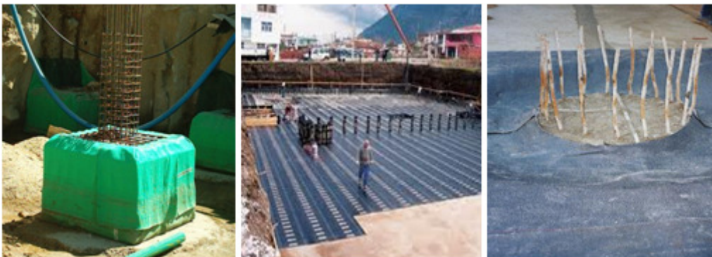
Figure 1 - Types of foundations that can be protected with waterproofing: isolated foundation footings, mat-slab foundations and pile heads [3] [w 1 ][w 2 ]
