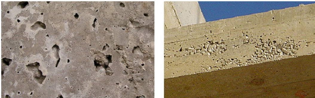
Figure 13 - Anomalies during execution: voids and segregation of concrete [w 4 ][w 5 ]
