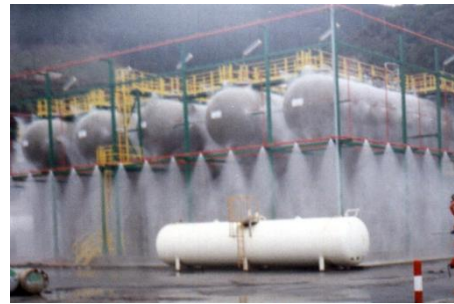
Image 2.6 - Water curtains system to protect tanks [12]
