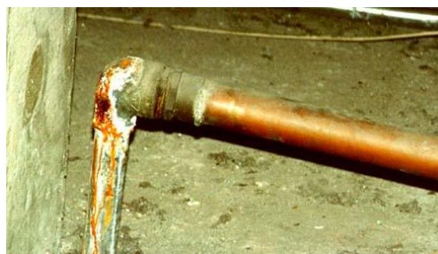
Image 3.1 - Corrosion in a metal piping [1]
