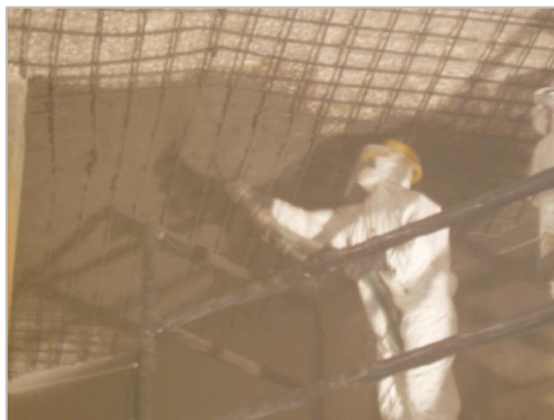
Figure 8 – Application of shotcrete on the bottom side of the top slab, which was previously reinforced.
