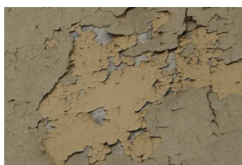
Figure 8 – Example of a “repaint over paint”.
