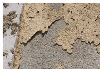
Figure 9 – Example of a “repaint removing paint”.
