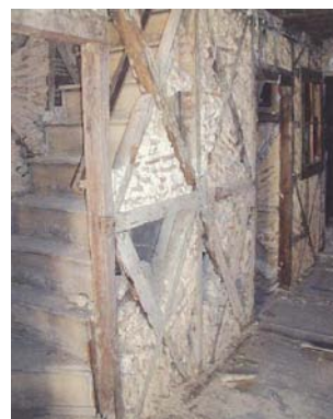
Figure 4 Frontal wall missing some masonry parts [APPLETON, 2008]
