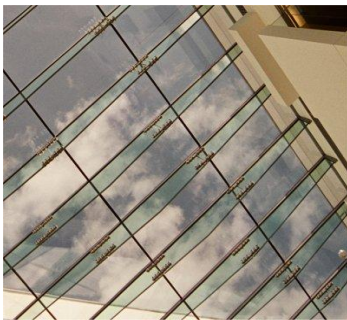
Figure 1 - Use of glass fins as support elements of a roof with a span greater than 15 m, Glasgow, Scotland [1].
