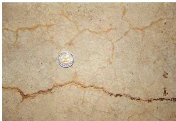
Figure 0.1 - Cracking type "craquelet" on the pavement of a dam crest (Silva, 2010)
