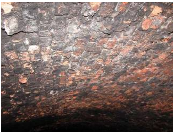
Figure 2 – Displacement and erosion of the masonry of the vault surface [2]
