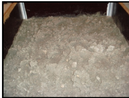
Image 8 - Aspect of the joint substrate surface obtained by the wire-brushing treatment
