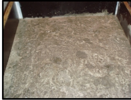
Image 7 – Aspect of the no treatment joint substrate surface
