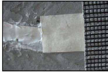
Figure 5: Local detachment of gypsum plaster and reinforcement with net ( R-D1 )
