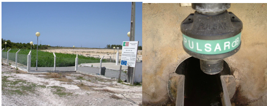
Figure 1 – Global view of Malavado WWTP and of the ultrasound transducer used to measure the flow.
