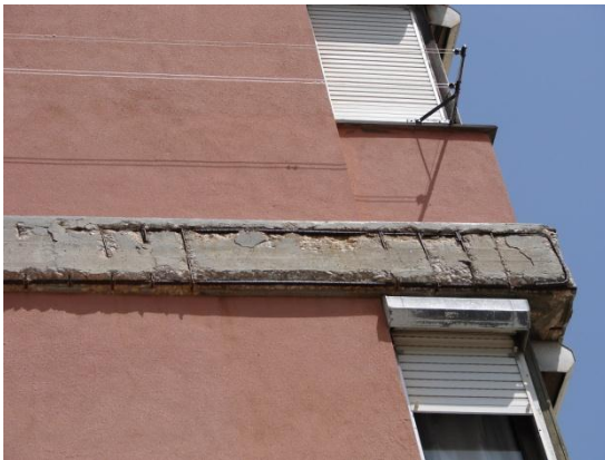
Detachment of the concrete cover and corrosion of reinforcement in beam
