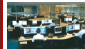
Control centre based on the SCATE X (Metro Do Porto, Porto, Portugal)
