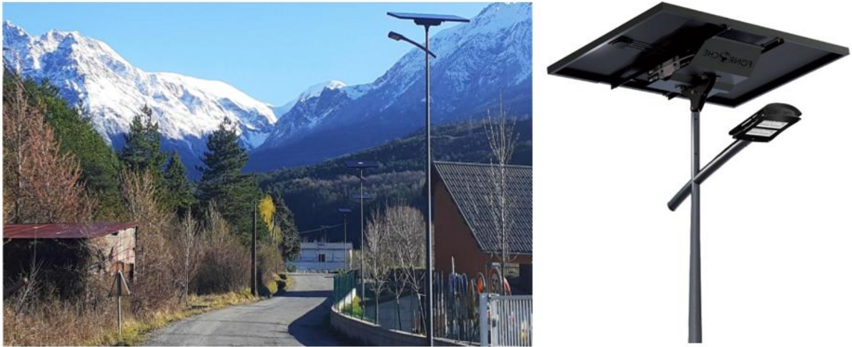
Figure 18: Solar street lighting in a French village 70 .
