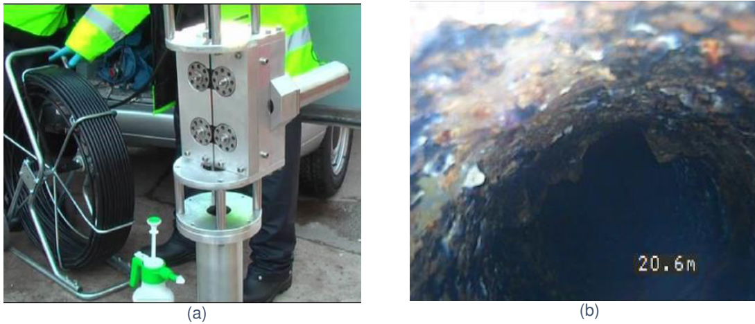
Figure 2-3 – Working CCTV camera system for condition assessment: (a) fire hydrant seal; and (b) controller view (API -Advanced pipe inspection UK Ltd., 2021).
