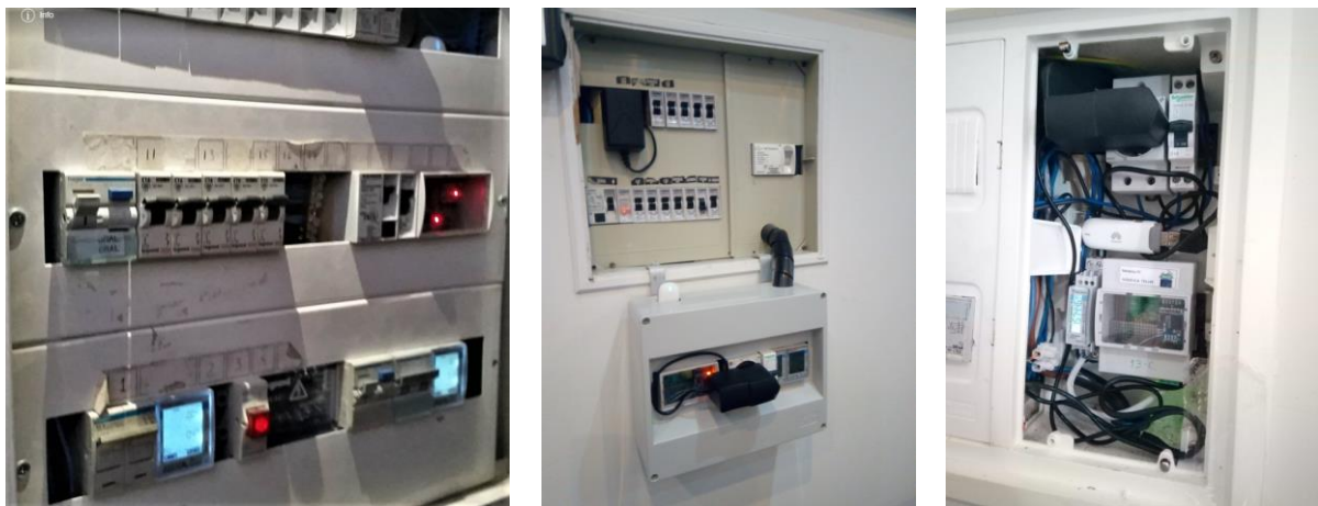
Figure 5.1 Examples of the Energy Monitoring System deployed in three UPACs
