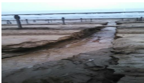
Figure 11: Cable trench slip due to rain
