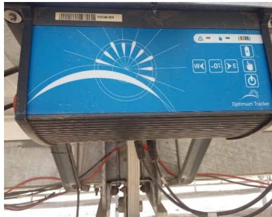
Figure 21: Tracker box communication issues rectified
