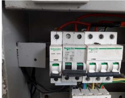
Figure 17: Fire alarm fault detected and repaired at circuit breaker level
