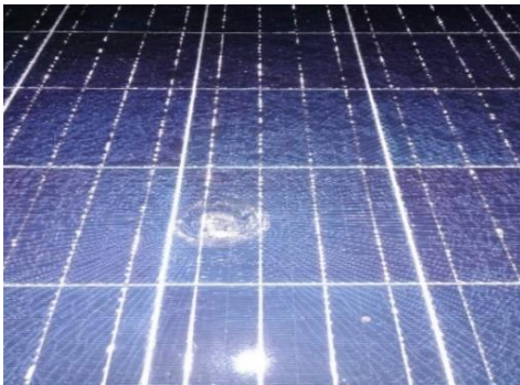
Figure 18: Damaged solar PV module
