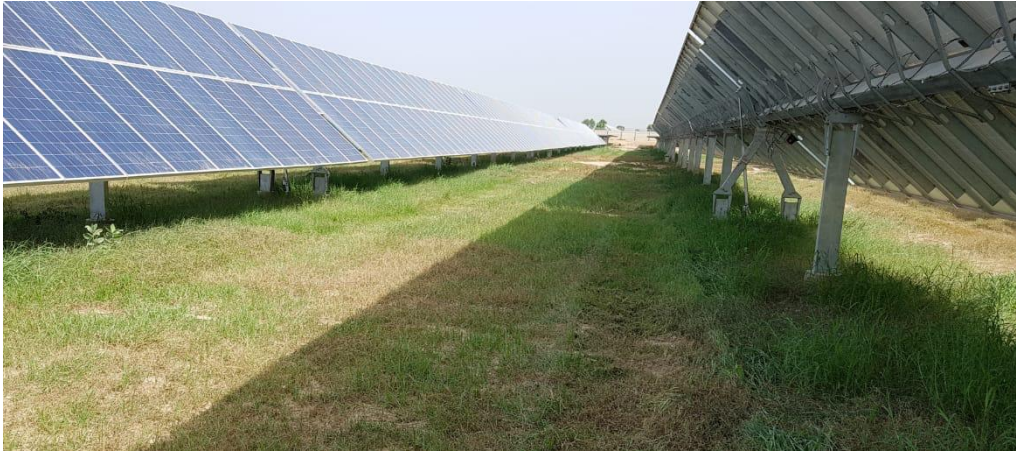
Figure 9: Rows of solar PV modules with 7 meters distance to avoid near shading
