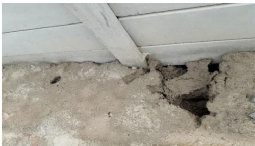
Figure 15: Boundary wall support soil displaced due to rain
