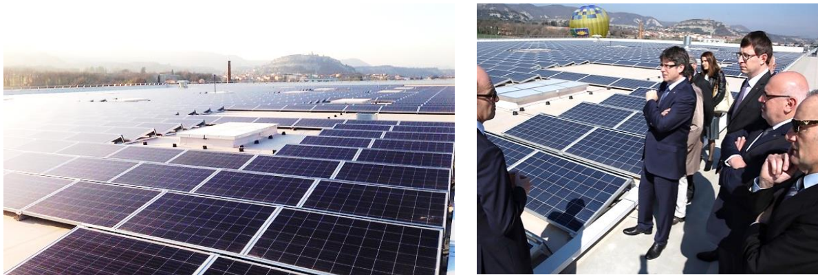
Figure 1. 650 kWp installation in the new warehouse of BonPreu, in Balenyà (Barcelona).
