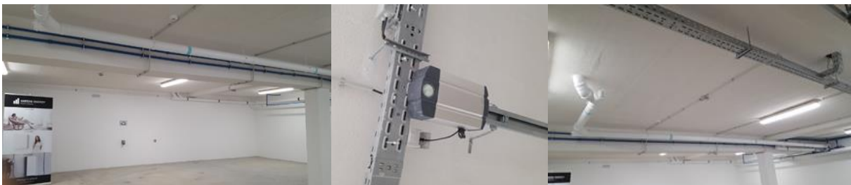
Figure 26. Parking area (left), garage door sensor (middle) and lighting systems (right)
