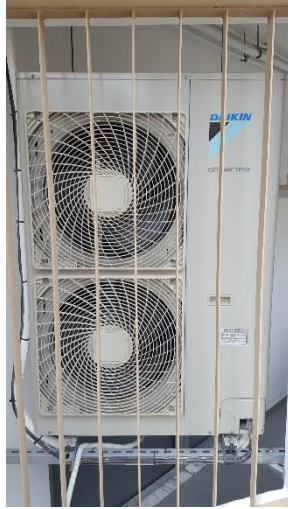
Figure 14. Daikin heat pump installed
