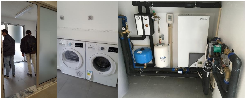
Figure 28. From left: view of the laundry room, energy efficient appliances, solar collector system components
