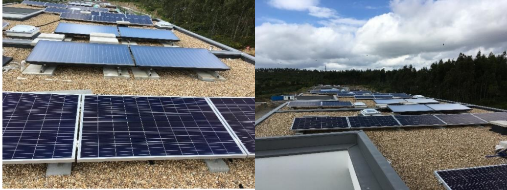
Figure 20. Spacing of collectors and PVs on rooftop (closer view)
