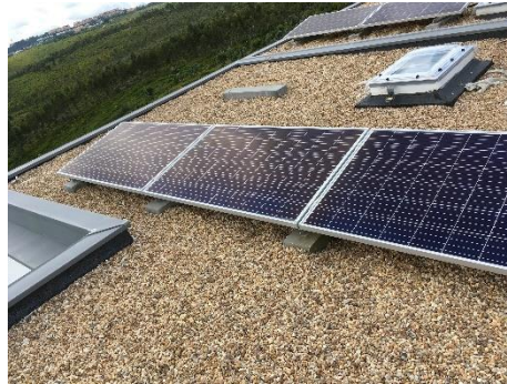
Figure 17. PV panel horizontal placement on rooftop
