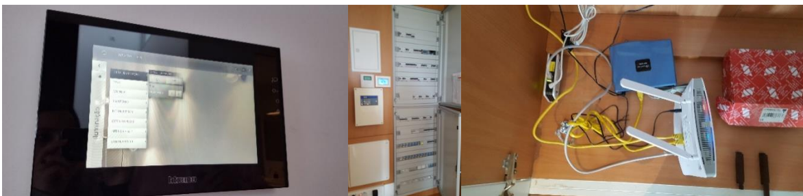
Figure 30. Domotics system panel, control panel and Wi-Fi modem
