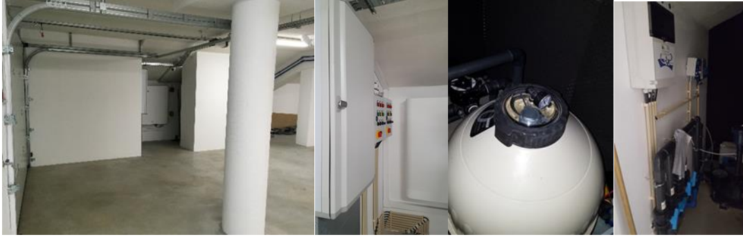
Figure 27. Main view of technical zone (left) and various installations
