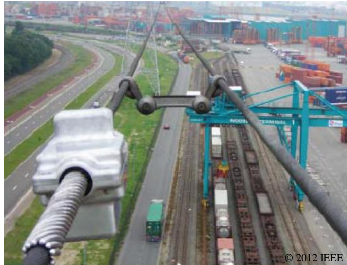
Figure 18: Ampacimon's device installation [38].
