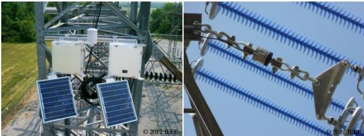
Figure 16: CAT-1 installation. PV panels are placed on the support tower to power the device [38].
