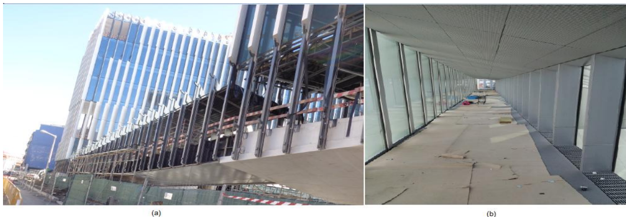
Figure 5.1-a) side view under construction and b) internal view after completion of the North footbridge
