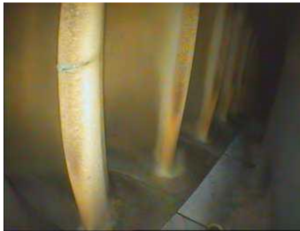
Figure 2.26 – Scratches on protective coating conducive to corrosion on the leading edge of a turbine blade. [49]
