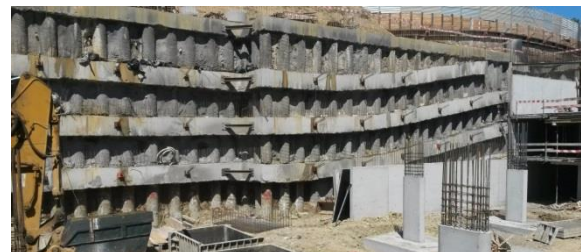
Fig. 5 - Bored pile curtain in the works of enlargement of Hospital da Luz's parking
